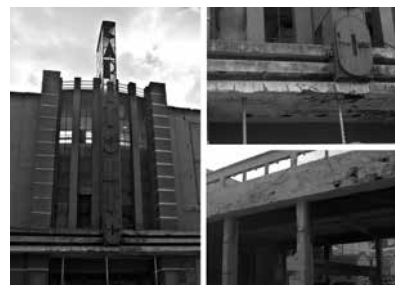
4. Decaying façade of Capit6lio (general view and details), Cristino da Silva 1931 © Joana Alves, 2010
